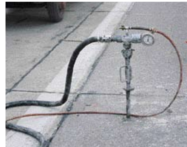
Here, the P 13 is seen raising carriageway slabs using a cement mortar.
